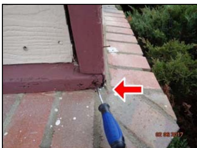
1.3 Item 1(Picture) Trim Next to Garge
