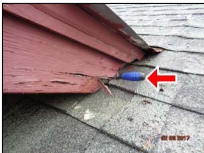
1.2 Item 1(Picture) Roof Rack Dry Rot
